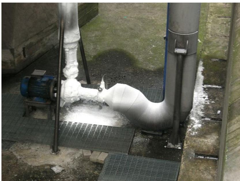
Pump fully covered with ice breaks down
