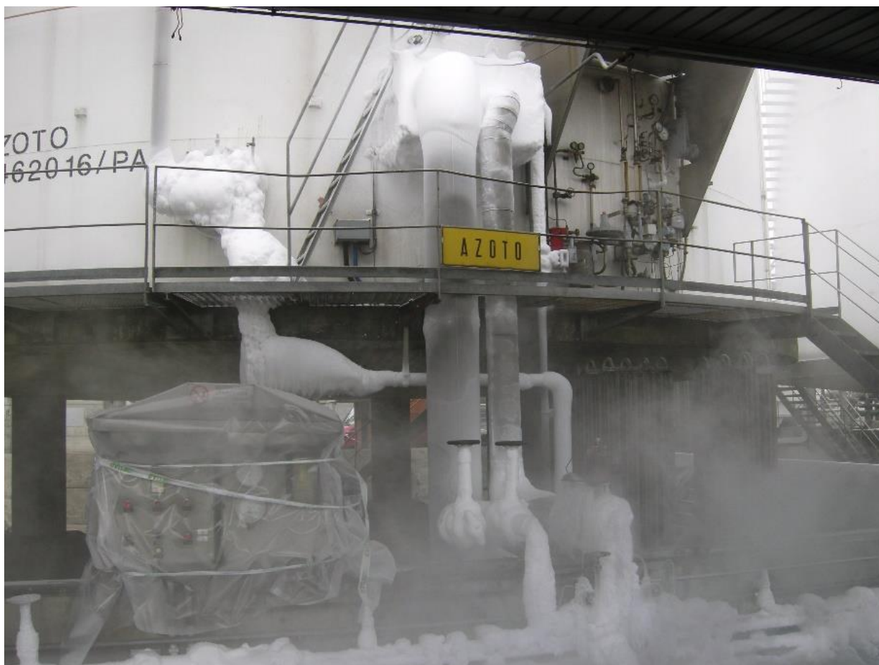
Control panel “protected” with plastic sheeting from the dripping condensation water. Extensive ice formation on pipes and valves
