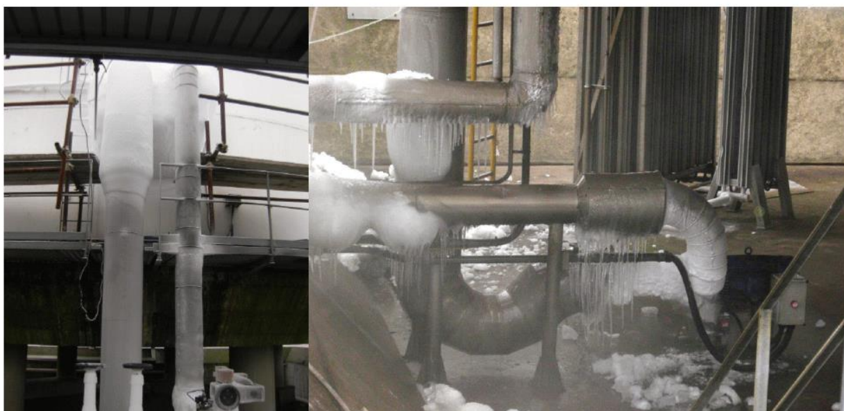
Broken vapour barriers and insufficient insulation caused ice to form around these pipes causing both process control and structural problems
